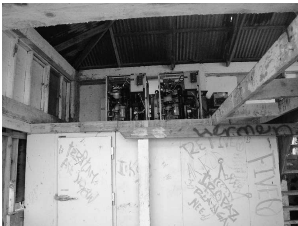
Fig. 7 A broken JICA ice plant (inside the plant).
